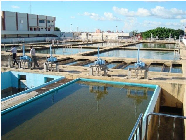
Water Treatment Plant, Cambodia
