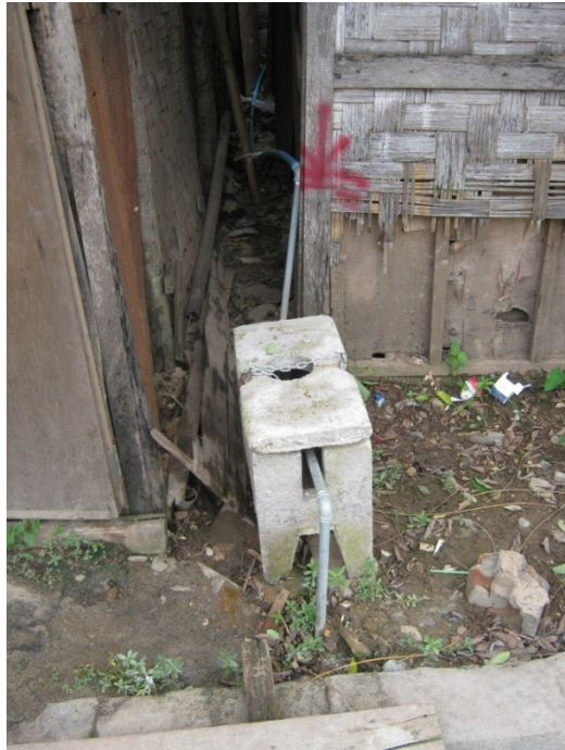
Connection to drinking water, Vientiane
