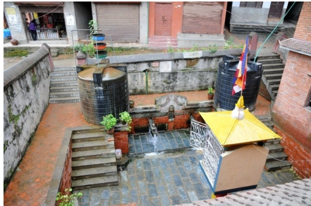
Drinking water purification plant, Lalitpur, Nepal
